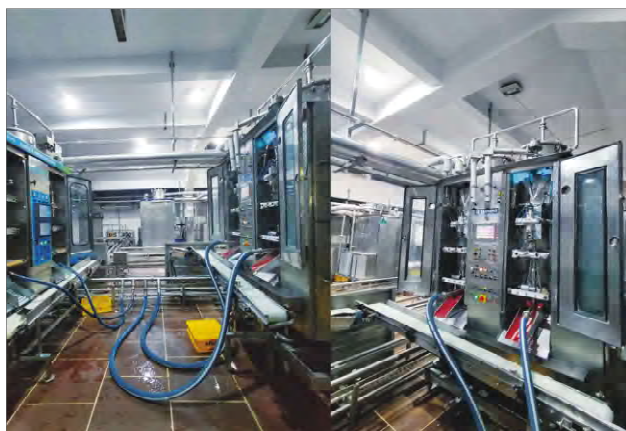
CIP Solution Recovery from Packing Machine
